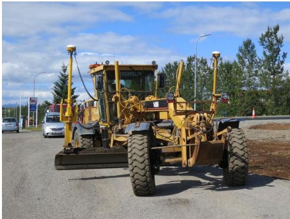
Figure 5.1 Grader with two GNSS antennas to control the blade. Picture (L. Steiner)
