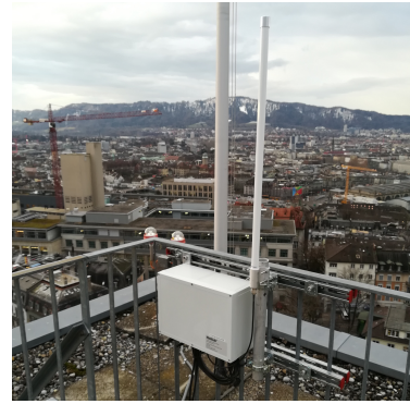
Figure 3: Rooftop node of FlockLab with high-gain antenna.
