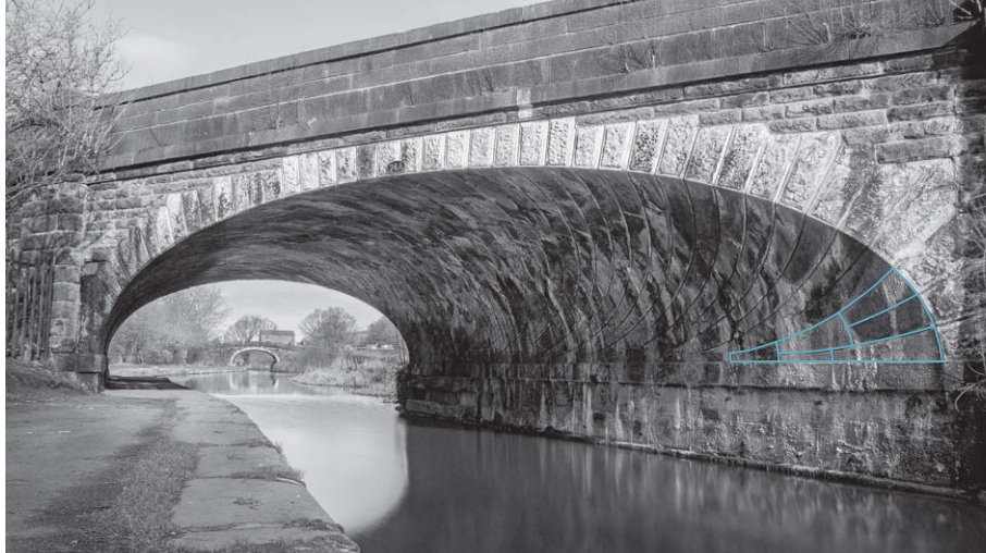
Figure 2.30: Bridge number 74A: Skew bridge carrying the Bolton and Preston railway over the Leeds-Liverpool canal, Chorley, United Kingdom (1840). Some intermediate voussoir courses near the abutments are traced in blue. (Image: James Perkins)
