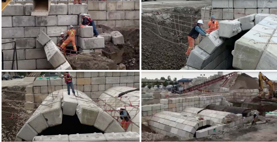
Figure 2.26: The assembly of a discrete barrel vault consisting of precast concrete blocks using the Arch-Lock™ construction system. (Image: Lock Block Ltd., 2008.)
