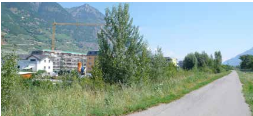
Construction site in the Rhône floodplain in Fully seen from the river levee (Rossano, 2013)
