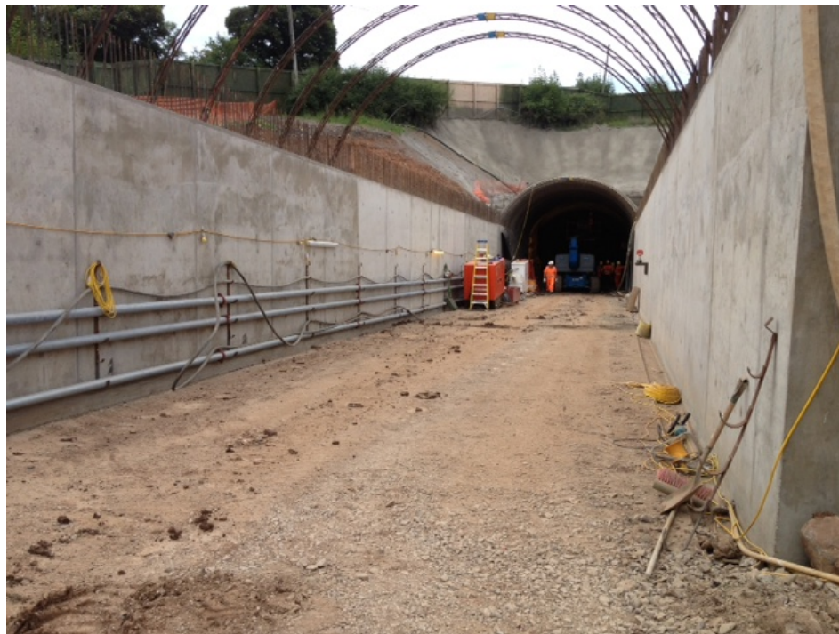
Fig 4: Newly-constructed (2013) entry to the mine, what is called an "access drift". (source: http://www.six-west.com/?p=902 )
