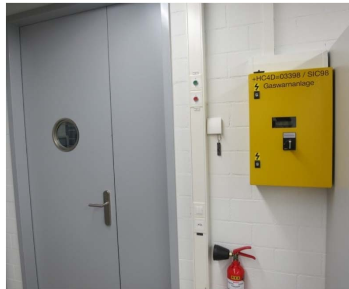
Wall-mounted control cabinet (yellow box) of the oxygen monitoring and alarm system in the MPMS3 lab
