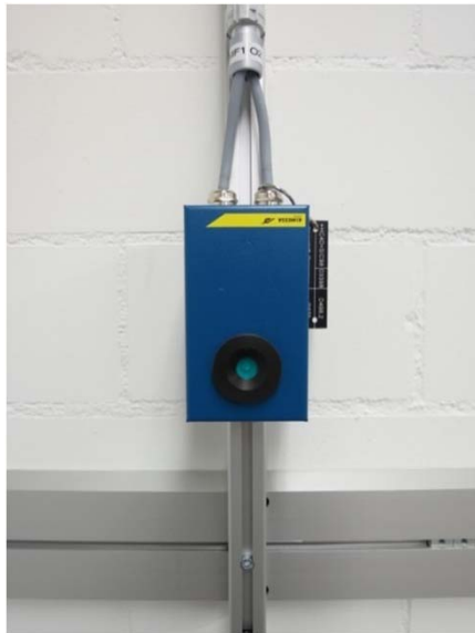
Wall-mounted oxygen sensor in the MPMS3 lab
