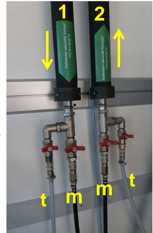
Cooling water port
