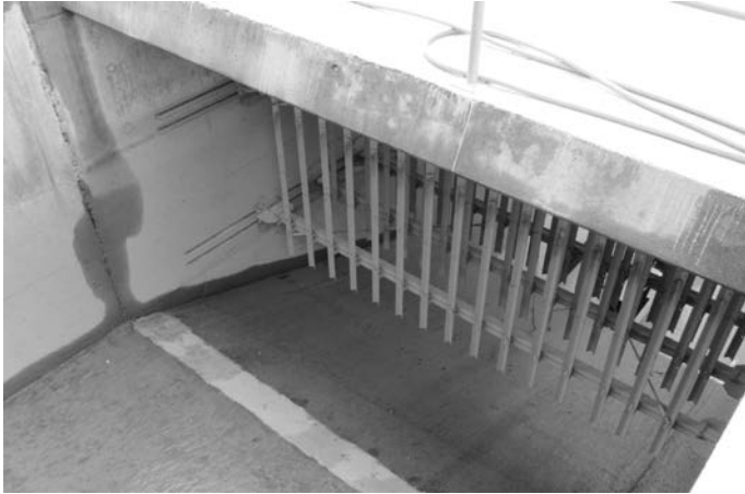
Figure 16. Three rows of tranquilizing racks with V-shaped bars (tips pointing downstream) upstream of the basin at Wysswasser. Source: VAW.
