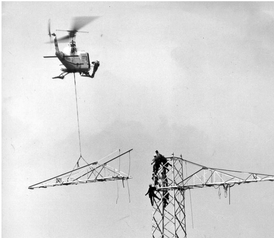
Fig. B.1: Aerial construction of a pylon with a Agusta-Bell 204B helicopter by Heliswiss (Walter Tschumi as pilot) in Sondrio, Italy, in 1969 [181].
