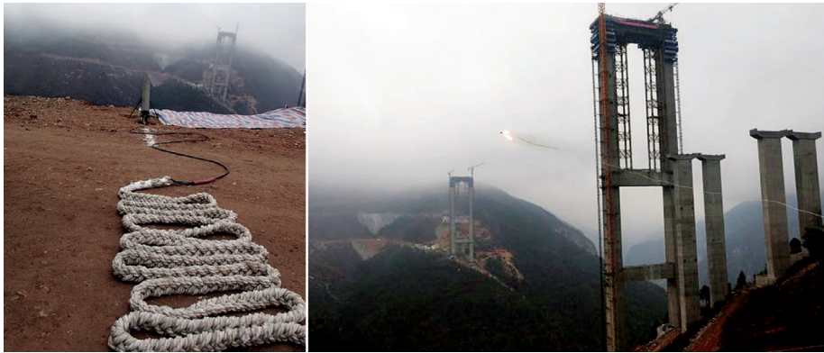
Fig. B.7: Tethered rocket for the erection of the pilot line for the main cable, in 2015, of the Puli Bridge in Pulixiang, China [196].
