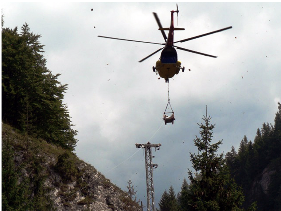
Fig. B.4: Helicopter stringing power cable in high-line construction. A worker stands on the pole to fasten the cable after the deployment. [189]
