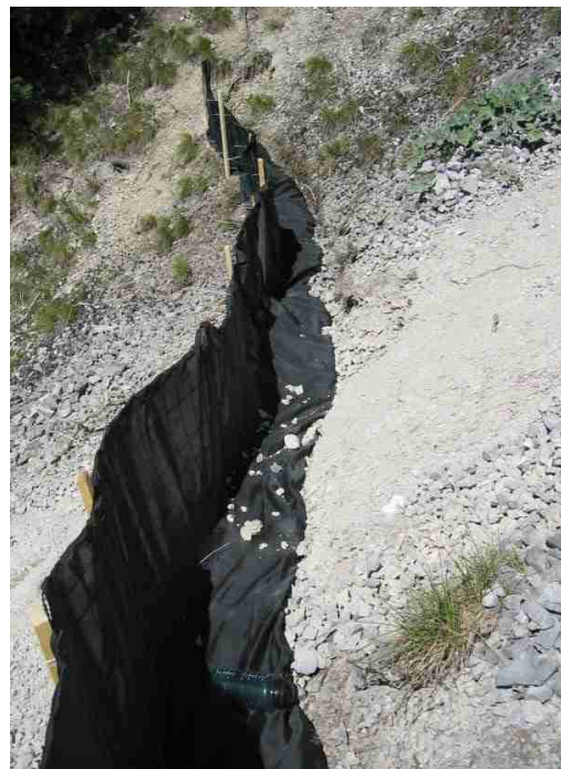
Figure 4-25 Silt fence plot G1 (Corina Gwerder)
