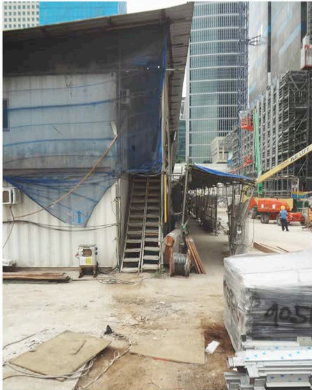
Dormitory on a construction site in Asia Square. Photographs taken during a clandestine visit.
