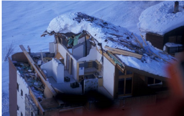
Fig. 1-7: Damaged house by an artificially released avalanche during the catastrophic avalanche winter of 1999 (Photo: J. Schweizer).
