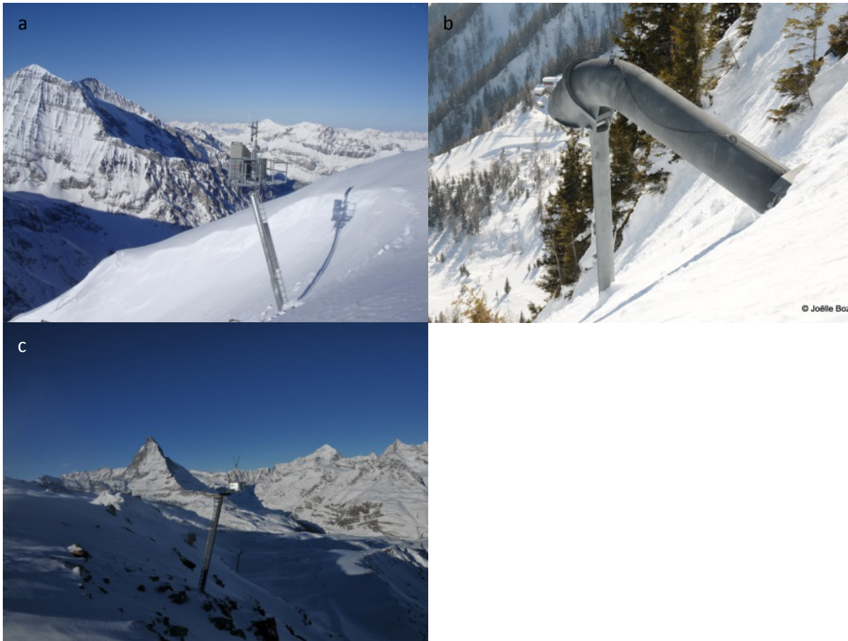
Fig. 1-8: Typical fixed avalanche release installations working with (a,c) solid explosives (SE) and (c) gas (DGE). Photos by Inauen-Schätti, Joëlle Bozon (TAS) and wyszen avalanche control.
