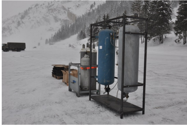
Fig. 5-2: Pressure reduction tanks for oxygen (blue) and propane (metallic). The gas bottles can be seen in the background.
