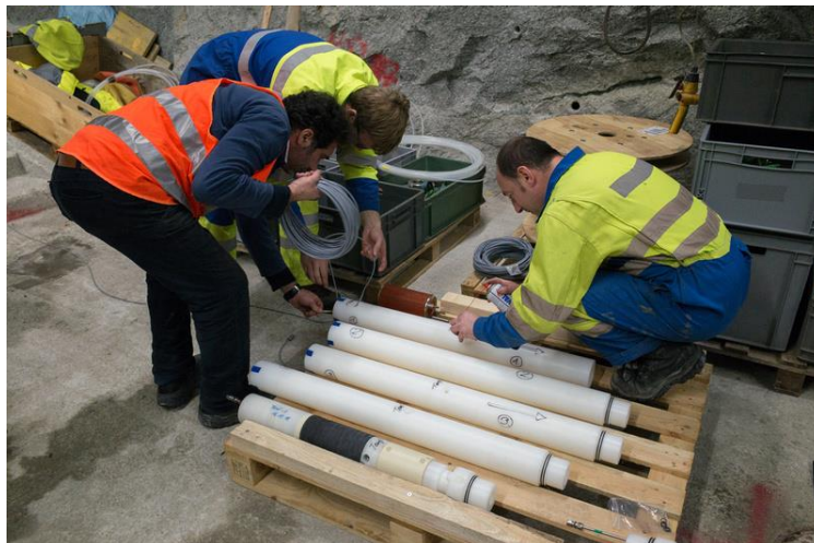
Figure B-14: PT1000 sensor installation at SBH 15.004 system (photo: H. Fisch, Nagra)
