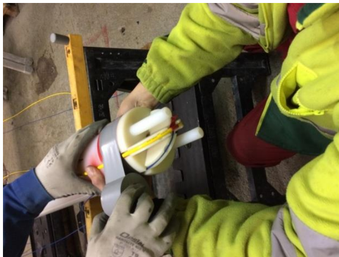
Figure B-2: Fibre optic cables fixed at system end
