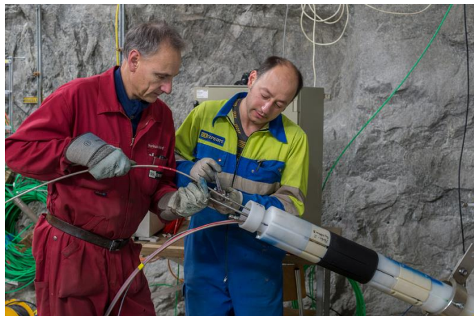
Figure B-11: Line tightness check during installation of PRP 16.003 (photo H. Fisch, Nagra)
