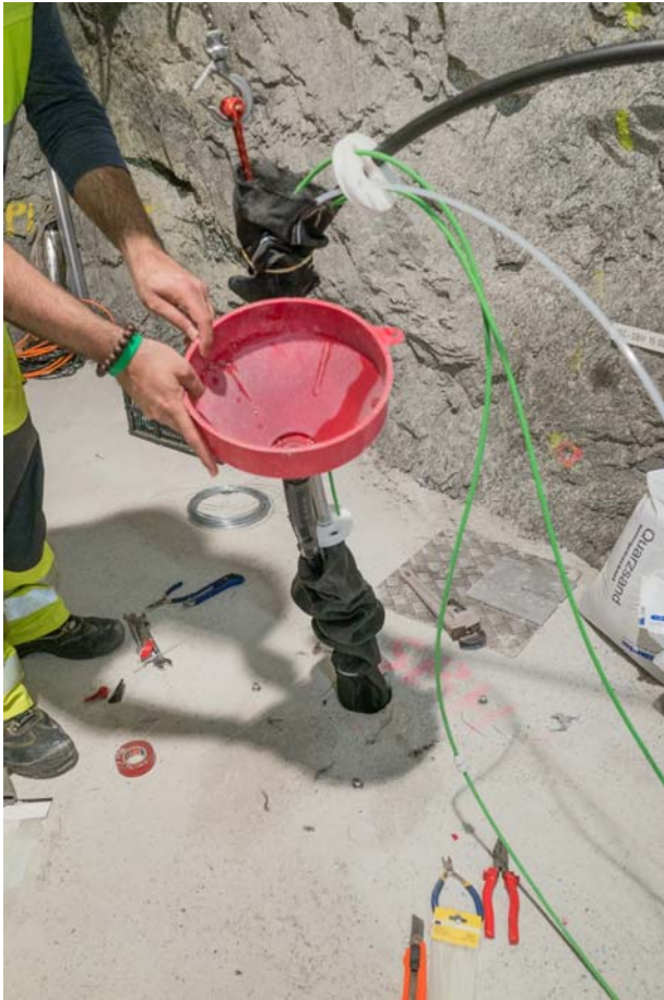
Fig. 4. Filing the geotextile sleeve of the central interval section with quartz sand.
