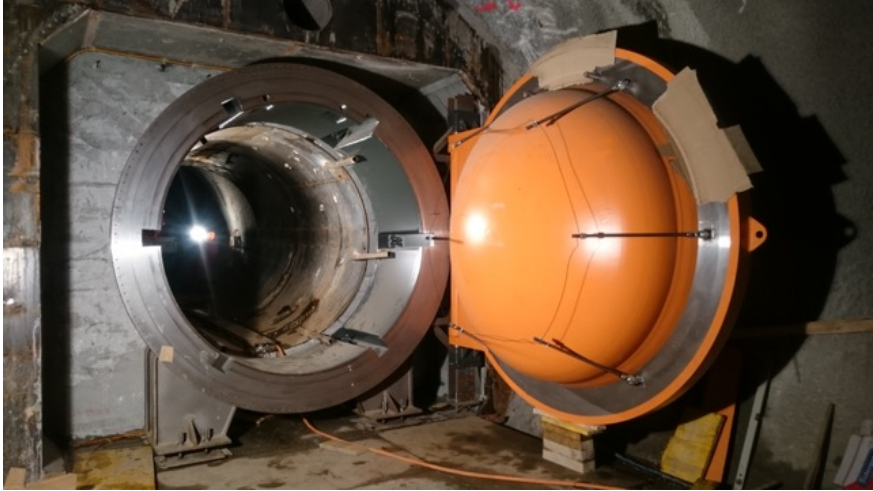
Figure 5.2: Picture of one of the concrete plugs and the associated steel door.
