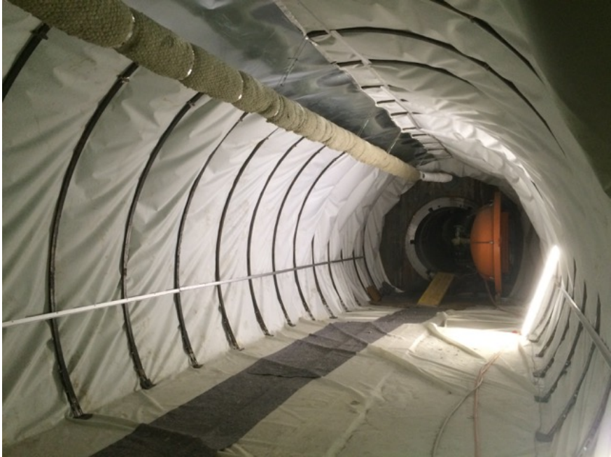
Figure 5.3: Picture of the impermeable high-strength glass-fiber membrane that was used to line the cavern near the concrete plugs. The insulated pipe through which the hot air enters and exits the cavern is visible at the top.
