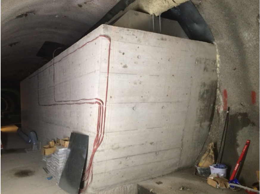
Figure 5.4: Picture of the TES inside the cavern. The red cables connect the resistance temperature detectors (RTDs) inside the TES to the data acquisition system. The positions of the RTDs inside the TES are shown in Fig. 5.5.
