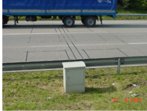
(B) Integrated road surface induction loops
