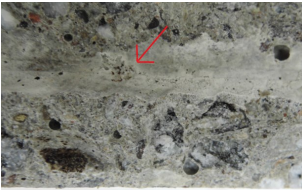
Fig. 3. Examples of irregularities at the SCI: Locally higher porosity (arrow) and small air voids (left part) as well as coarse air voids (right part). Corrosion initiated in this case at the arrow.
