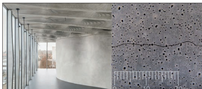
Figure 4: Finished concrete components of the DFAB House in Dübendorf, Switzerland. Left: Façade mullions fabricated by Smart Dynamic Casting seen on the left side (photo: dfabhouse.com ). Right: Shrinkage crack observed within days of fabrication of one of the façade mullions (photo: Thibault Demoulin )
