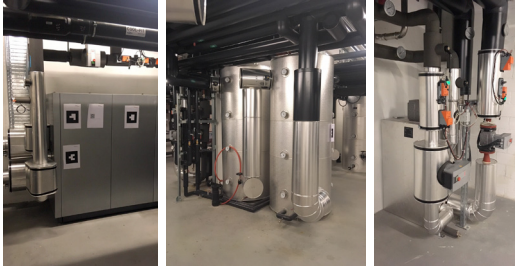
Fig. 3. Experimental set-up with heat pump, water storage tanks and heat exchanger
