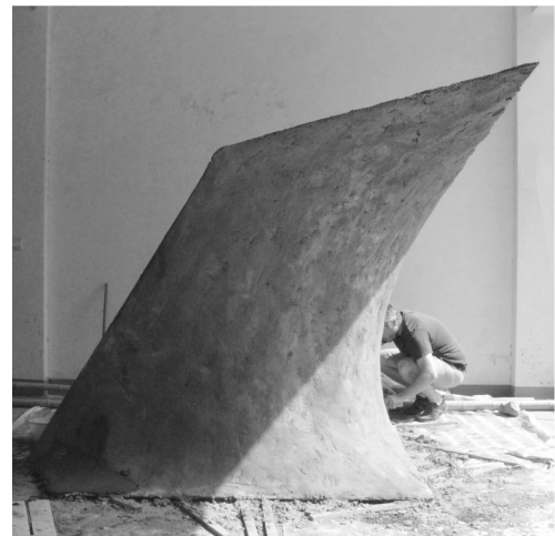
Fig. 18. A smooth poly-hypar surface made with ferrocement. Six hypar modules were welded from steel rebars, assembled into the skeleton of a cantilevering shell (above), wrapped by a steel mesh (middle), and then covered with concrete (bottom).
