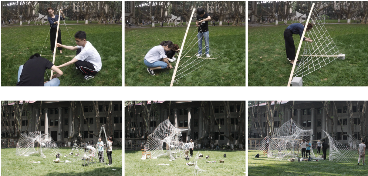
Fig. 15. Fabrication of one hypar with two wooden diagonals to keep four edges in the right position (above). Assembly of the pavilion (below) at the Southeast University of Nanjing (China).
