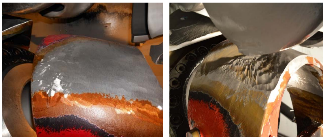
Figure D-20 Deflector of lower nozzle of MG 1 a) in original shape in April 2012 and b) with erosion in August 2012 after the major flood event.
