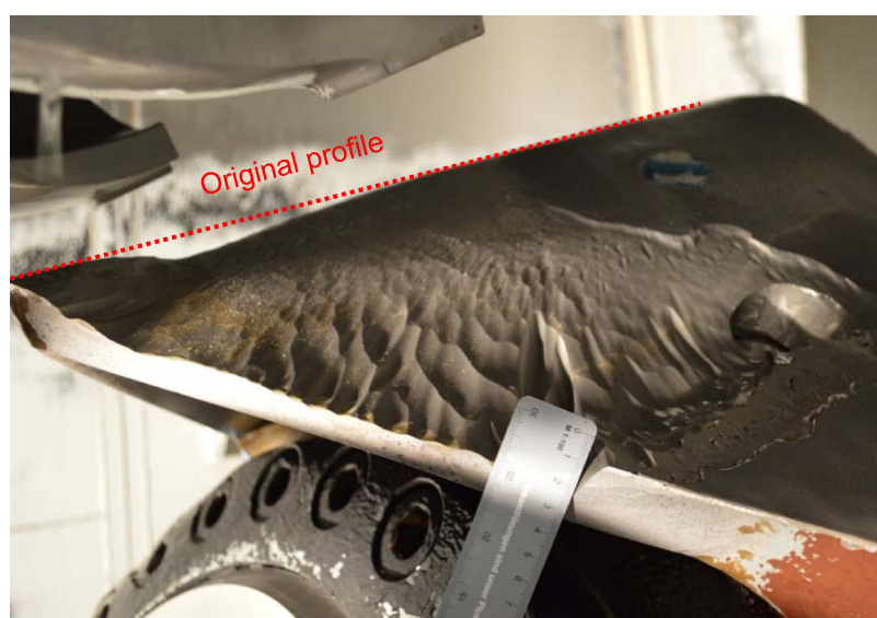
Figure D-21 Eroded shield of the lower nozzle of MG 1 in August 2012 after the major flood.
