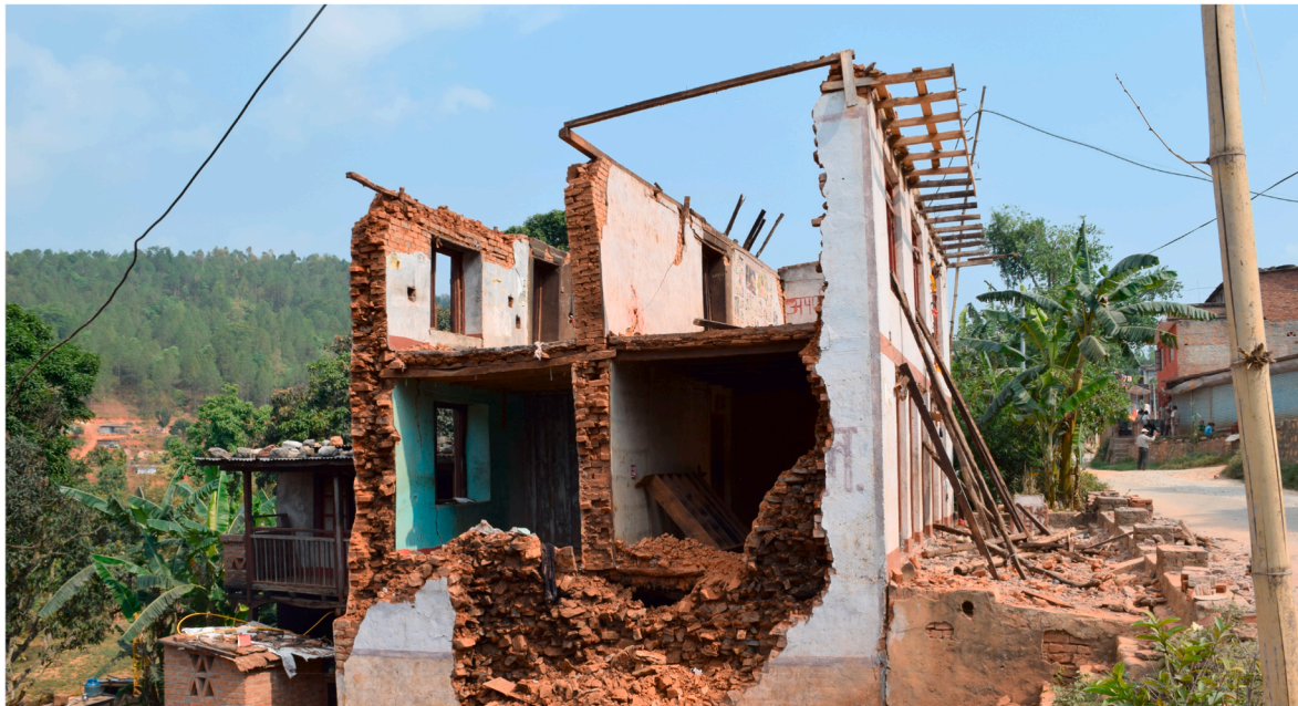
Fig. 17. Out-of-plane failure of brick masonry structures subjected to 2015 Gorkha earthquake (Credits: Dr. Rama Mohan Pokhrel).
