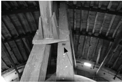
Figure 9. d02: topside of the upper collar-beam with the empty joint for the previous brace position (photo: author).
