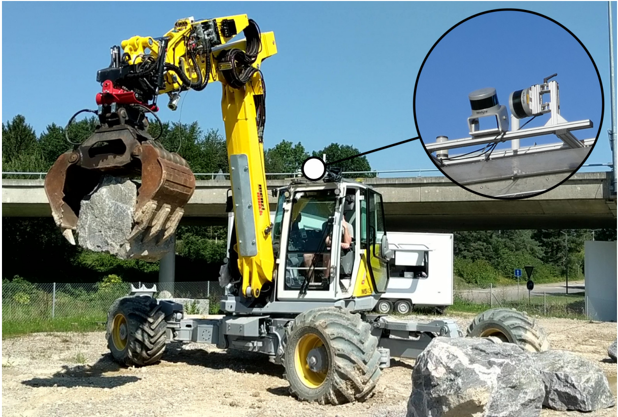
Figure 4.2: HEAP is an autonomous walking excavator based on a highly customized Menzi Muck M545. It is equipped with onboard sensors for state estimation ( GNSS , IMUs , and encoders) and scanning the environment (3D LiDARs ). As shown in the inset, the two LiDARs are mounted perpendicularly to each other such that a scanning motion is achieved not only while driving the robot around, but also while swinging the cabin.
