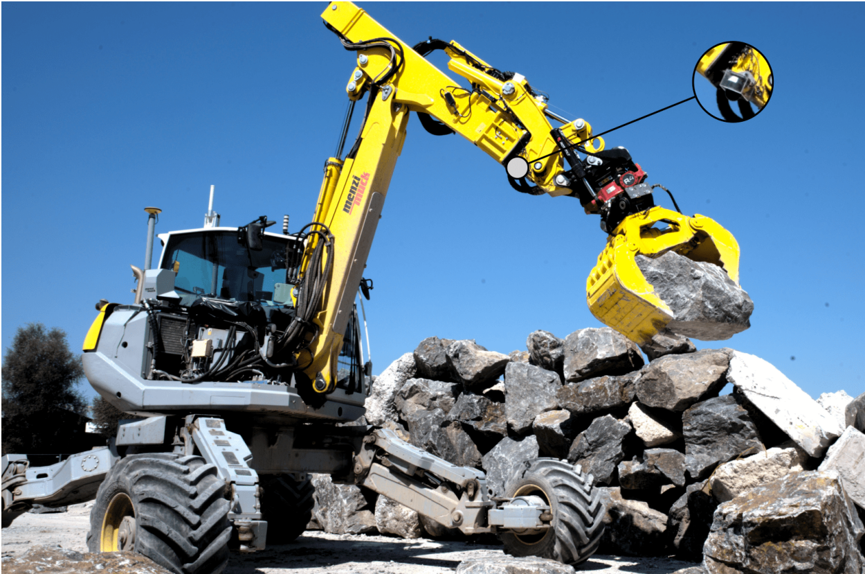
Figure 5.1: The autonomous excavator HEAP assembling a dry stone retaining wall with irregularly shaped stones. As shown in the inset, an arm mounted LiDAR is used for mapping and stone localization.
