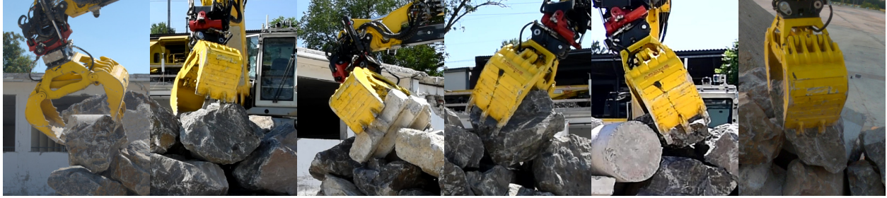
Figure 5.9: Examples of stone placements at the desired location. The placement grasps comply with the challenging collision constraints and enable to fit objects even in tight spaces.
