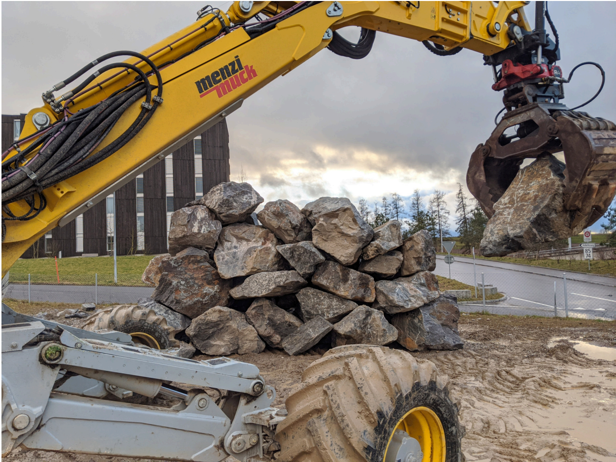
Figure 7.1: The stone wall constructed with the autonomous hydraulic excavator HEAP consists of 40 stones with masses between 230-1548 kg.
