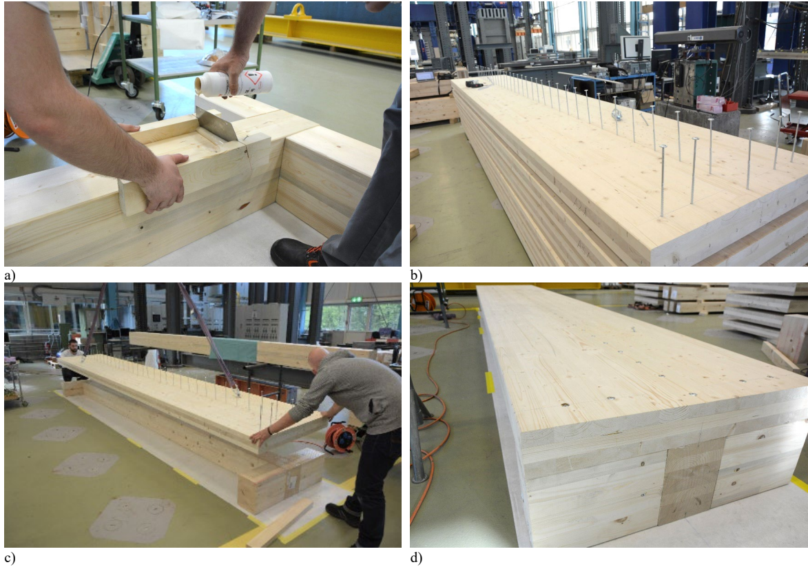
Figure 3.3. Reference tests - Screw-press gluing at ETH Zurich: a) Application of Purbond HB S709; b) Preparation of large washer head screws; c) Assembly of composite components; d) Assembled test specimen (minimum curing time: 175 min).
