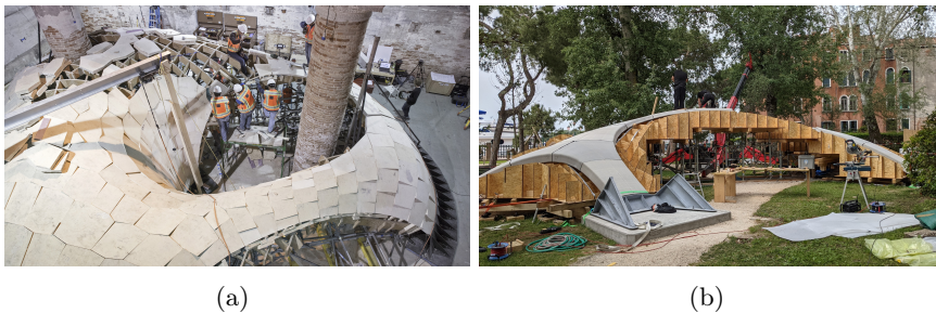
Figure 1.3: The construction and assembly process of (a) Armadillo Vault [Block et al., 2017c] and (b) Striatum [Bhooshan et al., 2022] require dense falsework.
