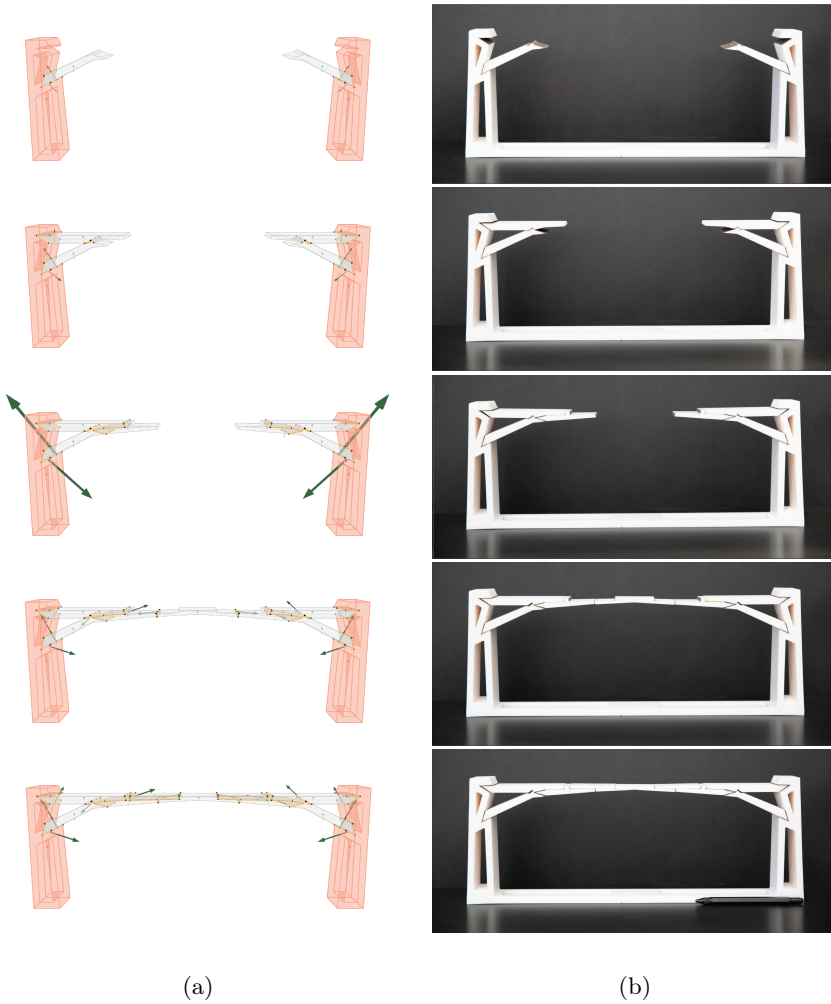
Figure 7.3: Sequential, scaffolding-free construction of the bridge. CRA analyses (a) and corresponding construction phases of the small-scale physical models (b).
