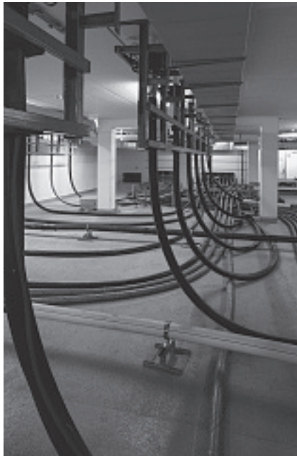
High-voltage cable room Photos: Tim Klausner
