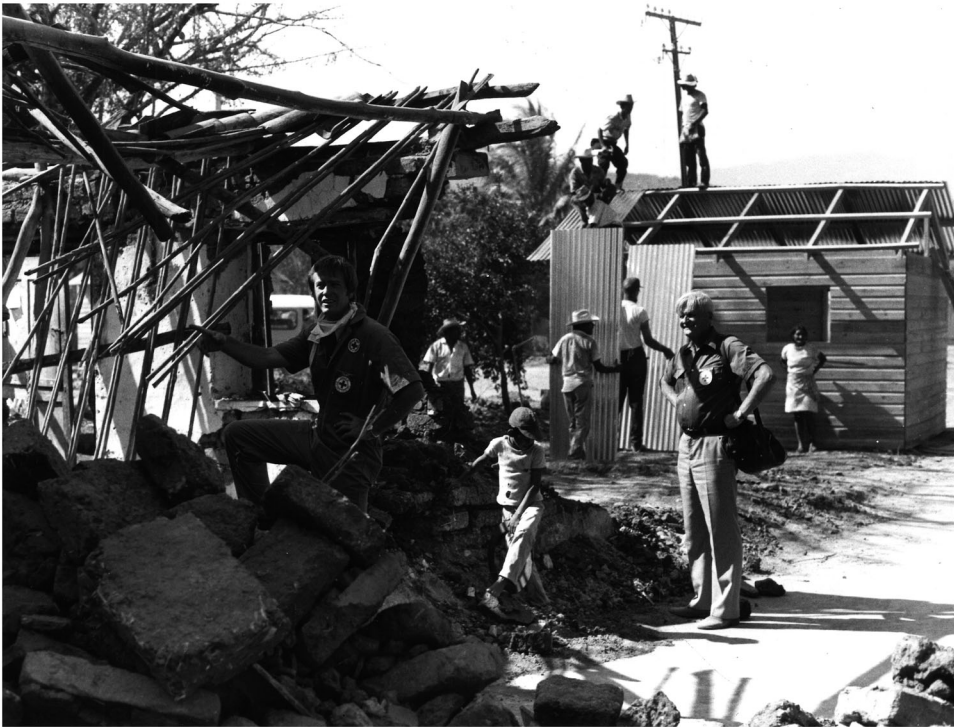
Figure 6. In the foreground, a destroyed house; in the background, a casita in El Progreso, built with materials provided by the Red Cross. The roof is being covered with corrugated metal sheets. Source: Swiss Red Cross Archives. The Swiss Red Cross (SRC) has made six images available for use in this academic article, depicting the intervention in Guatemala following the 1976 earthquake. The SRC understands these images to be free of rights and free of charge. The SRC is not aware of any third-party claims arising from copyright or licenses. It cannot, therefore, be held liable for any claims by third parties. Reuse is not permitted.
