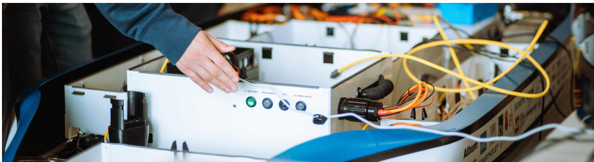
Figure 5.1: Battery box integrated into the prototype
