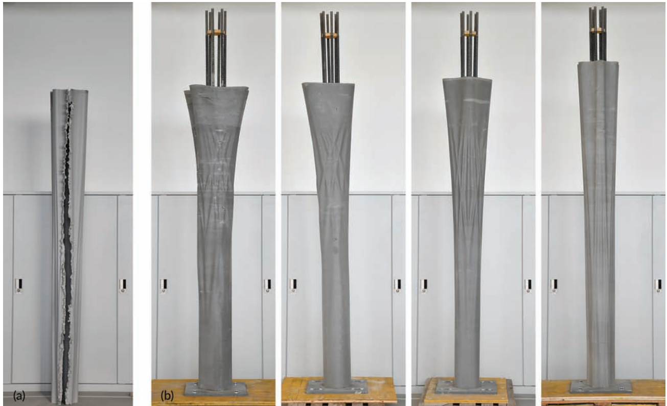
△ Figure 8. (a) One of the used column formworks printed with rPIPG, (b) the four cast and demolded columns of the Eggshell Pavilion.
