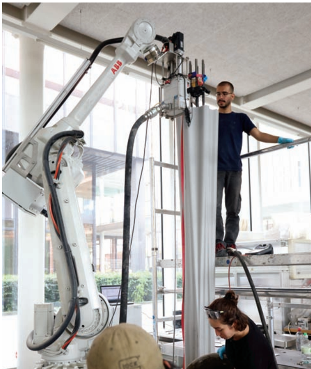
△ Figure 7. Fabrication process of the columns. (a) 3D printing process of one of the formworks—the other three formworks can be seen standing in the back, (b) filling the formwork using Digital Casting Systems.
