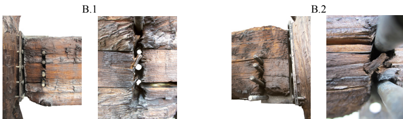
Figure 9. Connections B.1 and B.2 after the fire tests.
