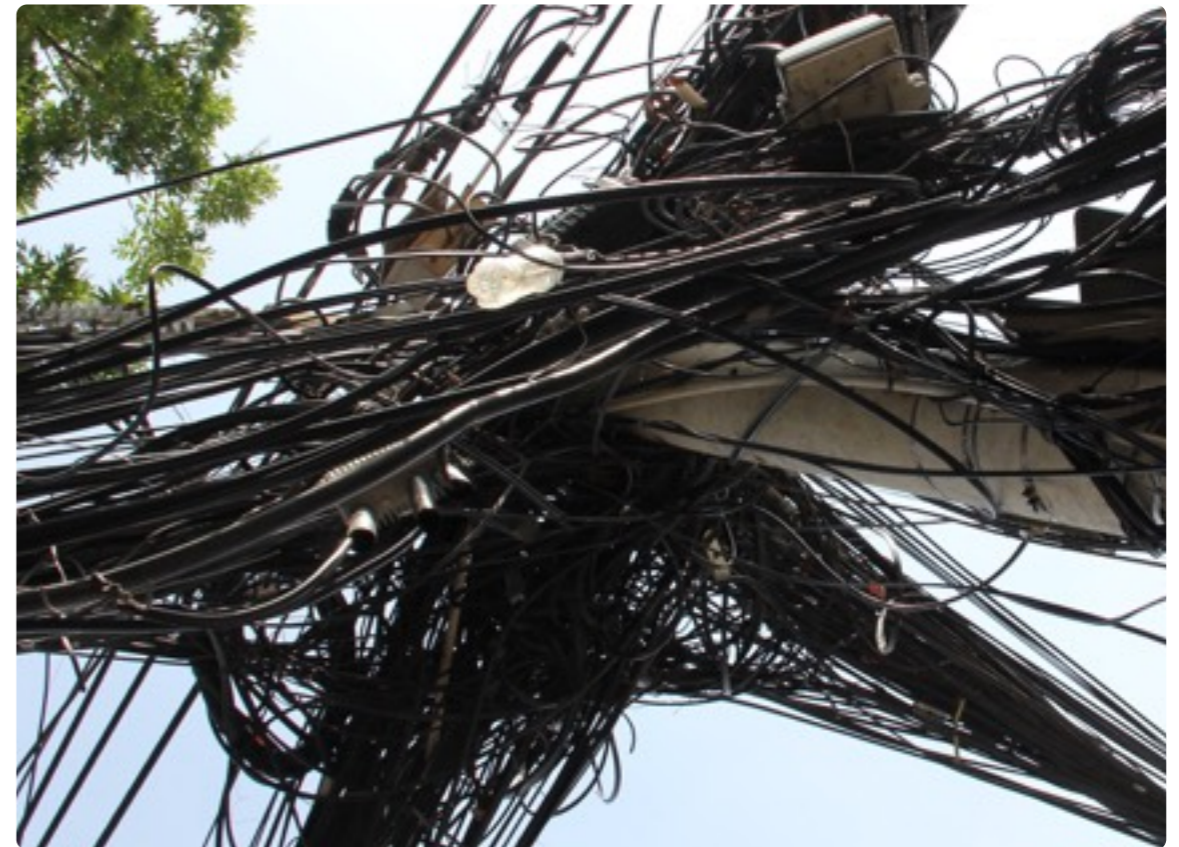
Bettschart, F. 2012. Electricity infrastructure. Multiple lines collect on concrete poles. [Photograph]. Ho Chi Minh City, Vietnam.
