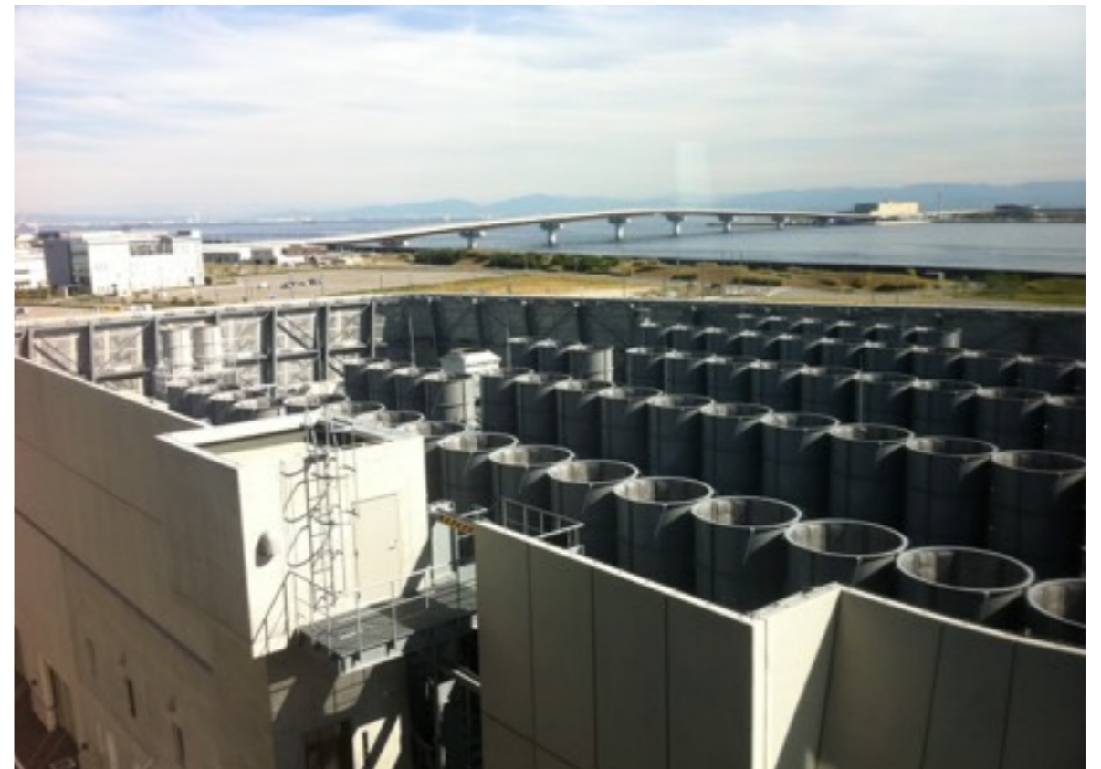
Schmitt, G. 2011. The K supercomputer in Kobe, Japan has an installed cooling capacity of almost 30 MW. [Photograph].
