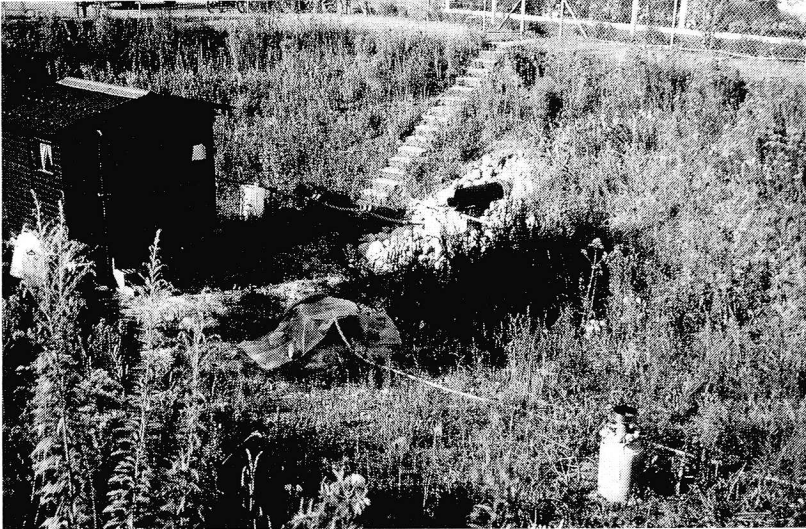
Figure 4.8 Storm water infiltration pit in Grütze with roof runoff inflow (black pipe) and sampling shaft.
