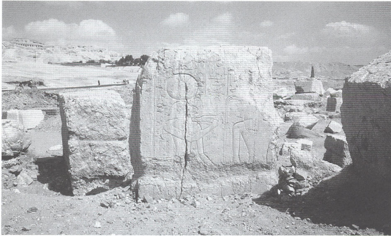
11. Blocks of decorated Qurna limestone showing a horizontal groove due to intense weathering just above the former air-soil interface. The base of the blocks has already been uncovered from debris for conservation.
