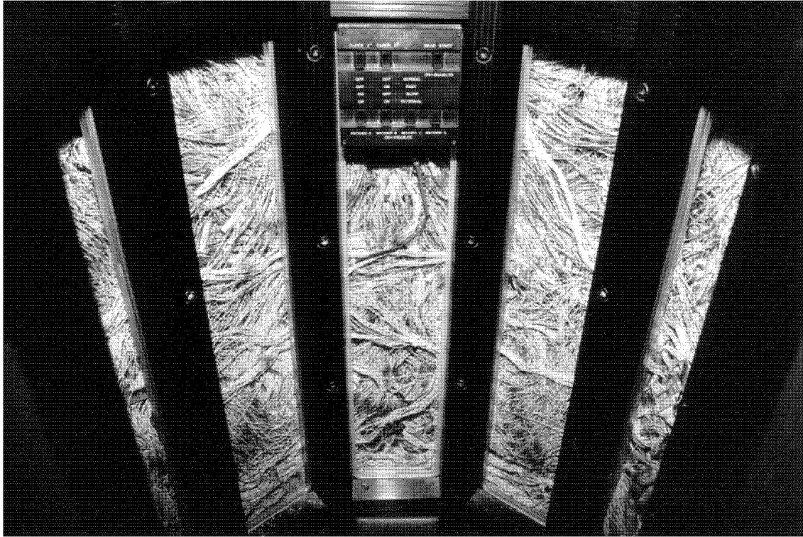
Figure 1.13: Internal wiring of the Cray Y-MP supercomputer
