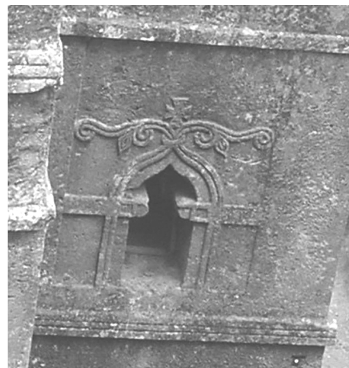
Fig. 2: Ornaments at upper windows and weathered corners of cornices in the foreground
