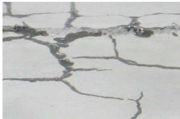
Fig. 2.24 Driven off water on the unheated side of a spalled element.
