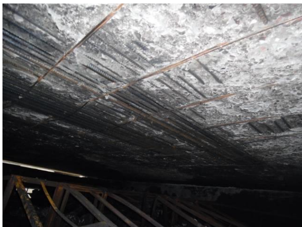
Fig. 2.4 Damaged element in the Wu Bridge (2015)
