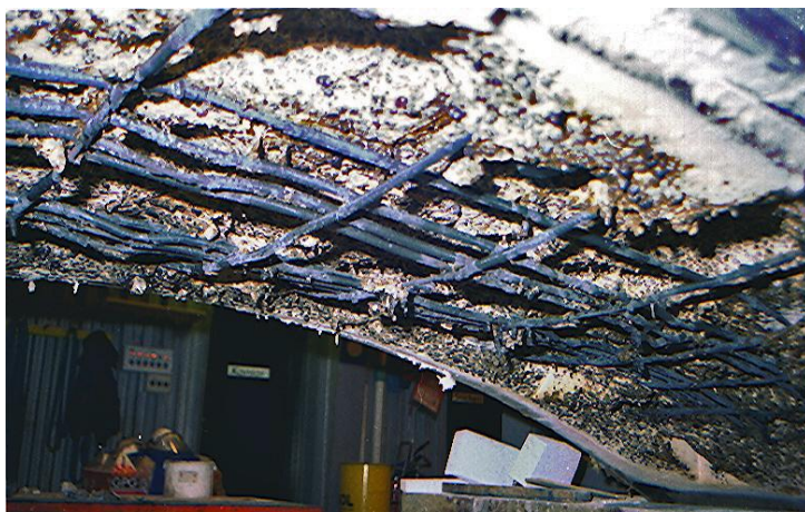
Fig. 2.1 Tunnel element from the Great Belt tunnel fire test at SP (Trafikministeriet 1995)
