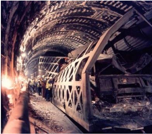
Fig. 2.2 Damaged section in the Channel Tunnel (Shuttleworth 1997)
