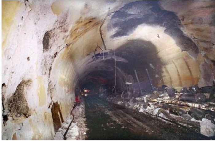
Fig. 2.3 Consequences of the Mont Blanc tunnel fire (Faure 2007).
