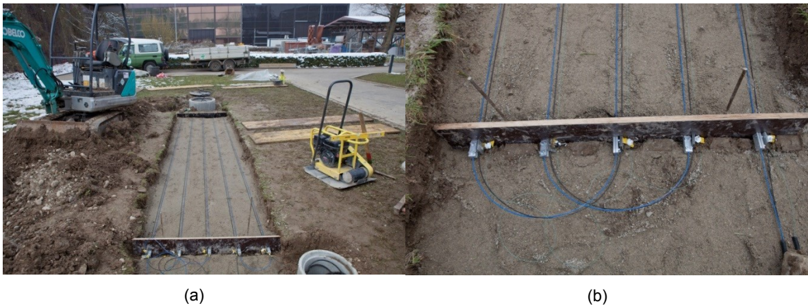
Figure 6-7. (a) Photo of the trench with pre-tensioned fibre-optic cables. Note, while here cables at a depth of 0.2 m are shown the presented experiment data is measured using FOS at a depth of 0.4 m; (b) Detail of the pre-tensioning of the FOS cables.
