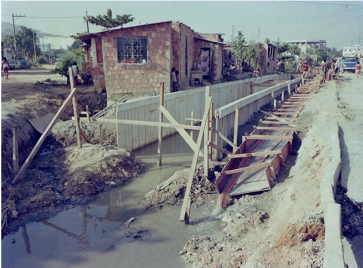
Fig. 2.42 Construction of a drainage channel in the suburbs of Rio de Janeiro. Lelé redesigned the system (1986) on the basis of the previous experience in Salvador. Photograph by Celso Brando. Arquivo Zeca Franco, Rio de Janeiro
