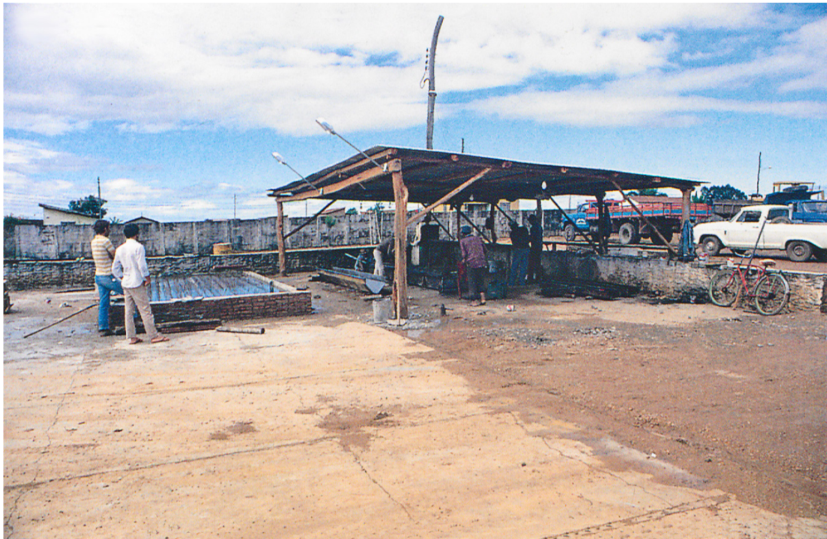
Fig. 3.32 First factory in Abadiânia to produce precast elements in argamassa armada . Implemented by Lelé in 1983, the factory was created to produce the small bridge's components. Arquivo João Filgueiras Lima, Salvador
