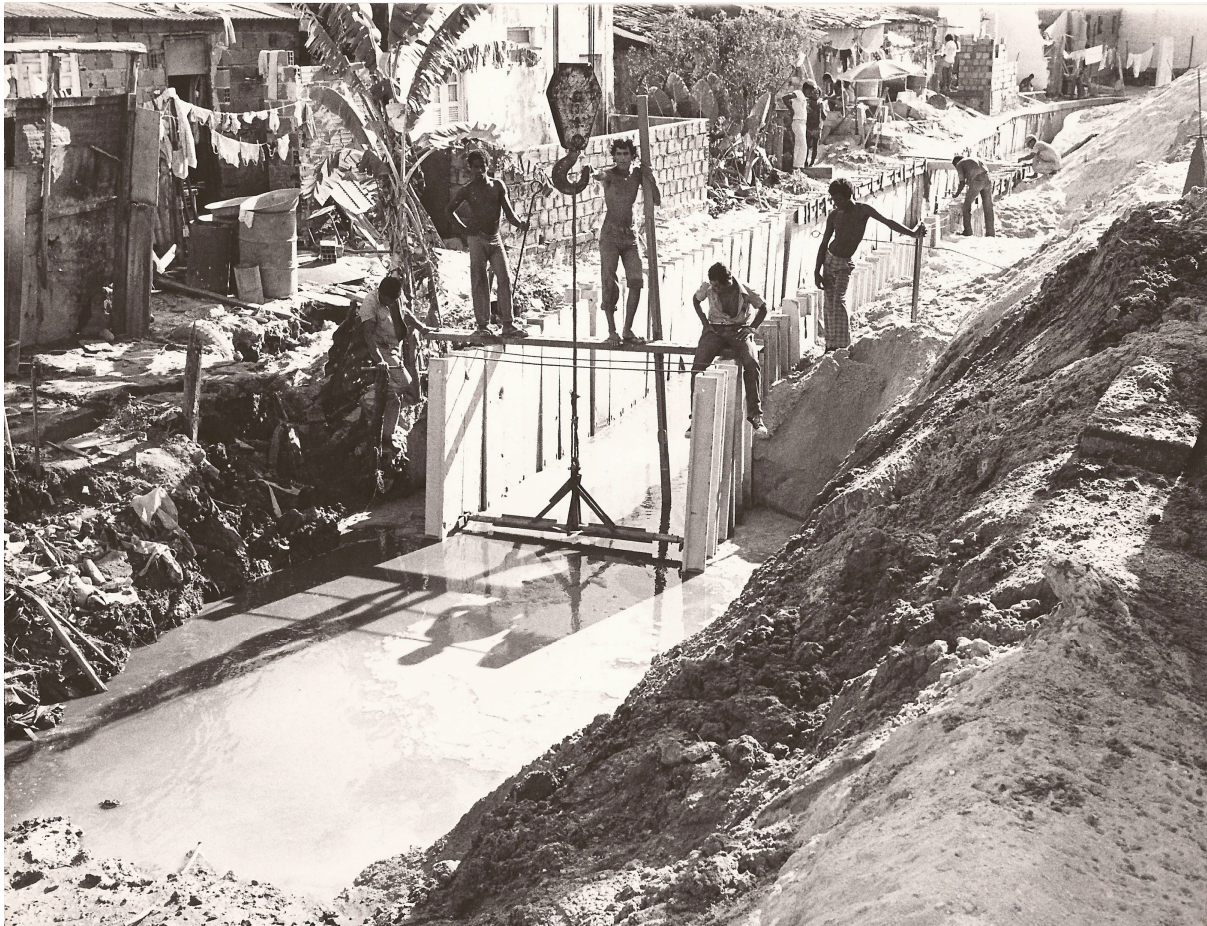
Fig. 3.24 Precast sanitation channels' assembly in progress on the outskirts of Salvador (1980). The articulated metallic bar allows the Munck truck to raise one triple module at a time. Arquivo Kristian Schiel, Brasília
