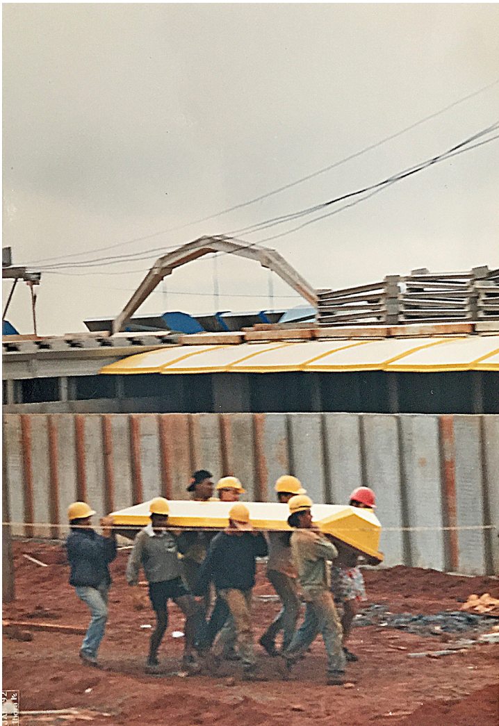
Fig. 2.97 Workers carrying the CIAC's sun-canopy in Brasília (1992) during the assembly of the first prototype. Arquivo Kristian Schiel, Brasília
