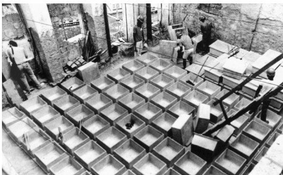
Fig. 1.8 Prefabricated slab molds. G. Latorraca, João Filgueiras Lima, Lelé (Lisboa: Blau, 2000), p. 167
