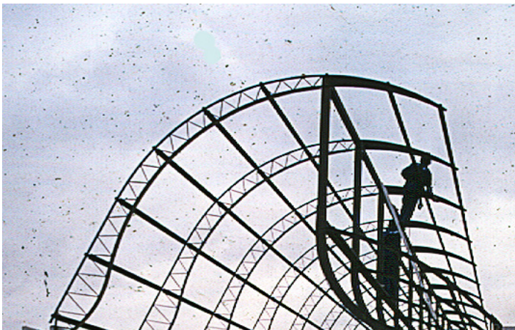
Fig. 2.106 Children's Rehabilitation Center. Roof trusses under construction. Sarah Hospital at Pombeba Island. João Figueiras Lima, Rio de Janeiro, 2001. Arquivo João Figueiras Lima, Salvador
