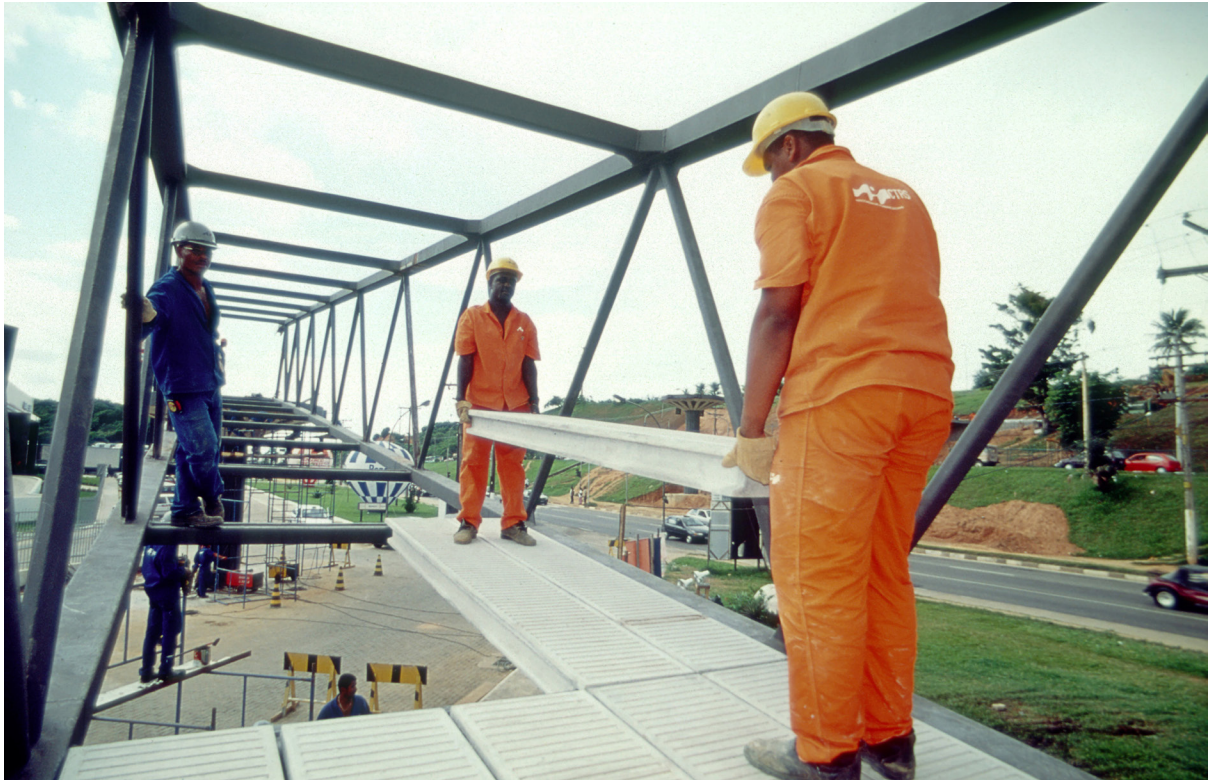
Fig. 3.74 Assembly process of the Pernambuco footbridge in Salvador showing the diagonal elements of the metallic truss. Lelé, 1986-88. Arquivo CTRS, Salvador. Courtesy of Waldir Silveira
