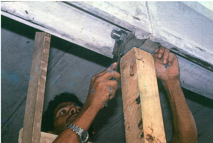
Fig. 2.63 The gutter-beam ( viga-calha ). Abadiânia, Lelé, 1982. A local worker joins the two halves of the beam by tightening the galvanized bolt. Arquivo João Filgueiras Lima, Salvador
