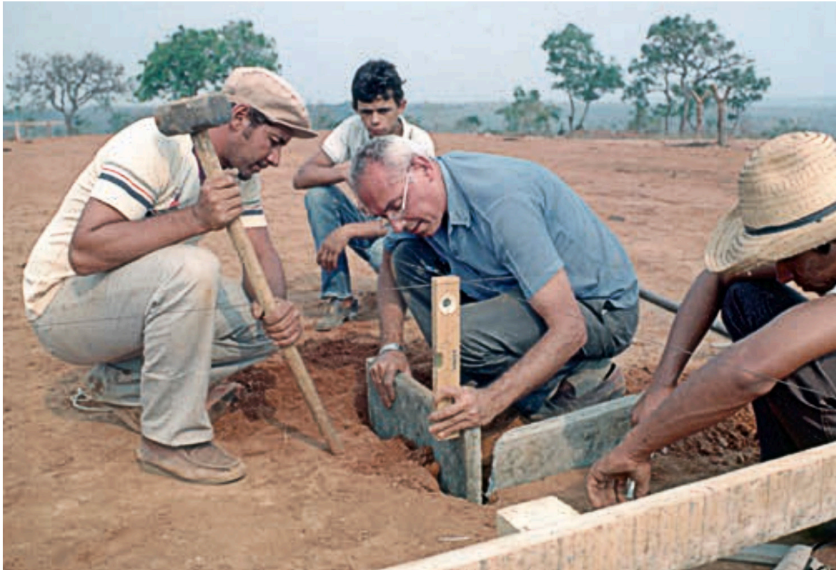
Fig. 2.46 Lelé supervising the start of building works in Abadiânia. Photograph by Mariana Chama. Marina Mange Grinover, PhD diss., Universidade de São Paulo, 2015, 382
