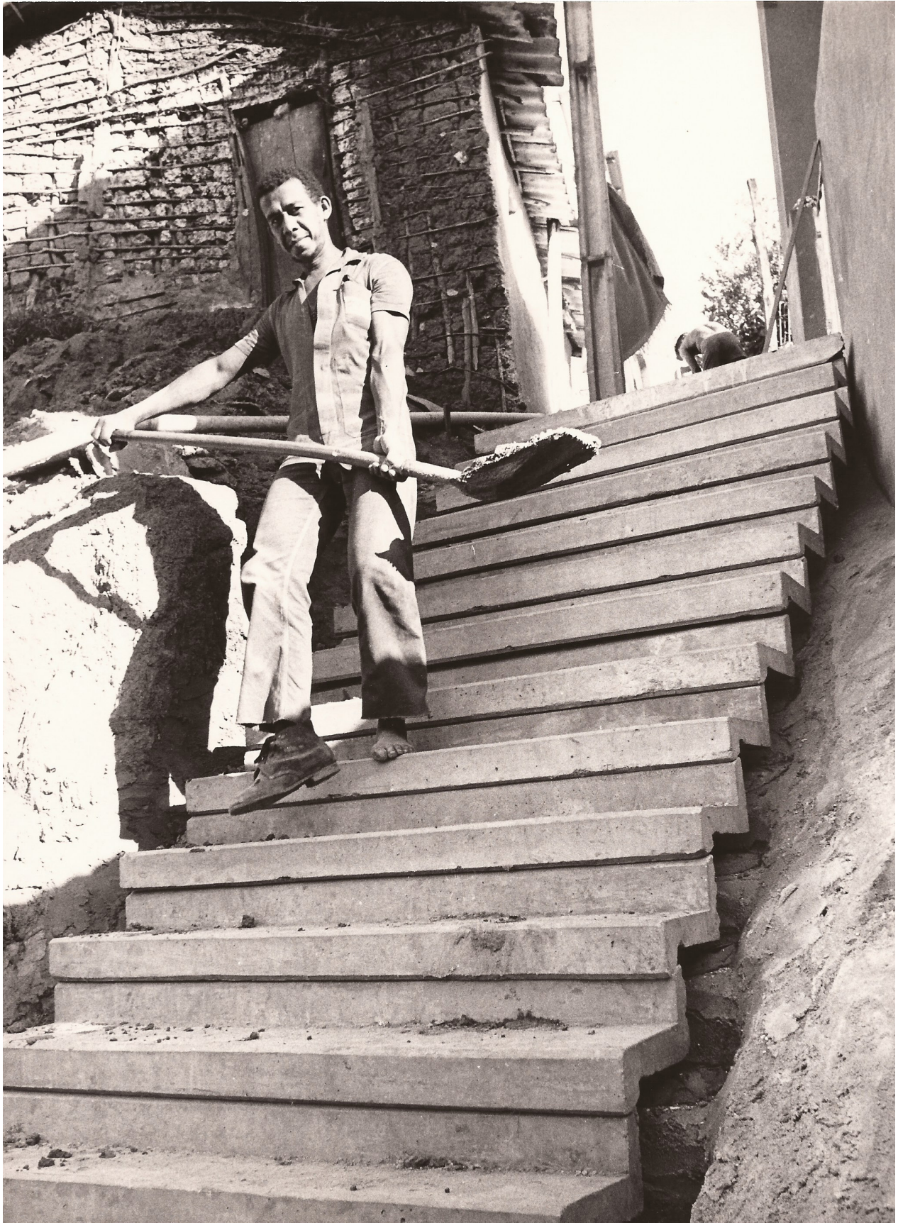
Fig. 2.1 Worker and local resident during the construction of prefabricated stairways as part of the sanitation project for the Camurujipe Valley in Salvador, Brazil (1980-81). Arquivo Kristian Schiel, Brasília
