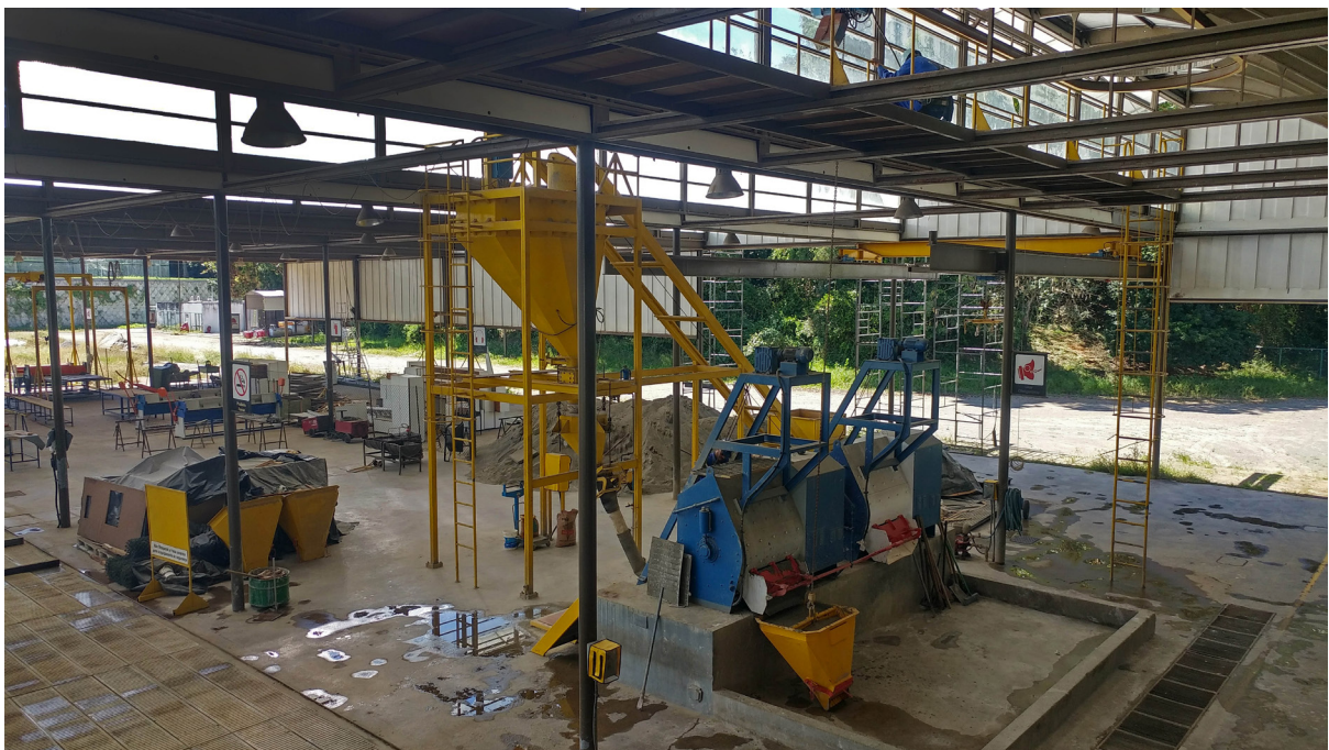
Fig. 3.73 The CTRS's argamassa central mixing plant. After the mixture is prepared, the argamassa is dumped into the yellow hoppers and lifted to the casting area. Photograph by Akemi Tahara, 2017. Courtesy of José Fernando Minho
