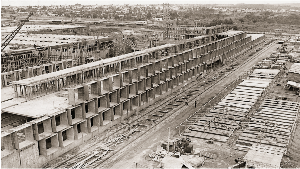
Fig. 1.51 Taguatinga Hospital's internment block under construction. The cast-in-place rigid central core is distinguished by a great amount of propping. Arquivo Kristian Schiel, Brasília
