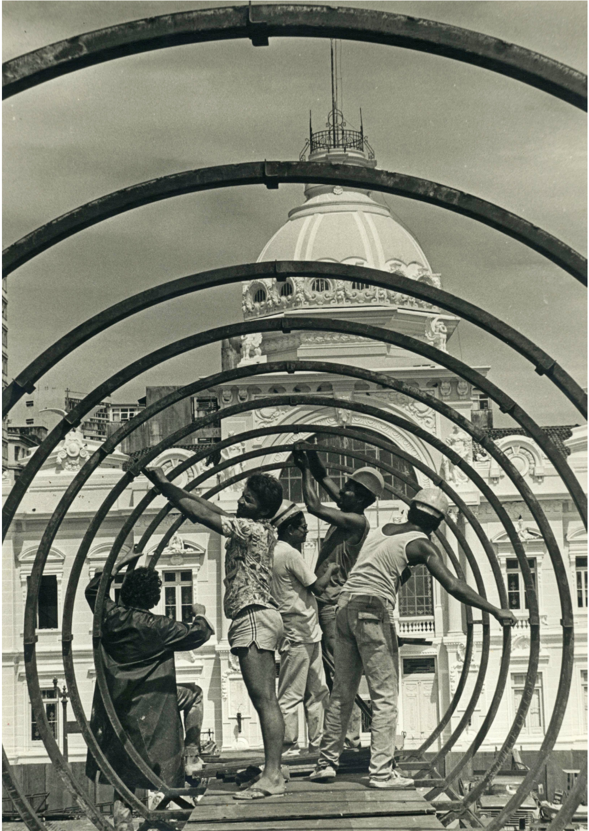
Fig. 3.1 Workers assembling the air conditioning duct on the roof of the Salvador City Hall (João Filgueiras Lima, Mariano Casañas, Roberto Vitorino, José Fernando Minho, and Emilia Emiko, 1986). Located in the city's historic center, the metallic structure was assembled in only 12 days. Fundação Gregório de Mattos, Salvador
