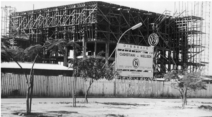
Fig. 1.39 Disbrave building under construction. João Filgueiras Lima, 1965. Arquivo Disbrave. Source: Audrey Migliani, Clássicos da Arquitetura: Disbrave . Archdaily, January 2015
