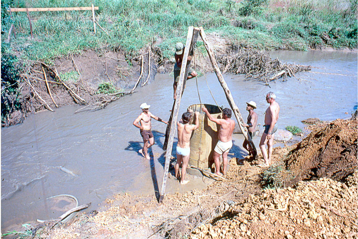
Fig. 3.25 Lelé (on the right) and the manual excavation works for the small bridge over the Curralinho river in Abadiânia, 1983. Arquivo João Filgueiras Lima, Salvador
