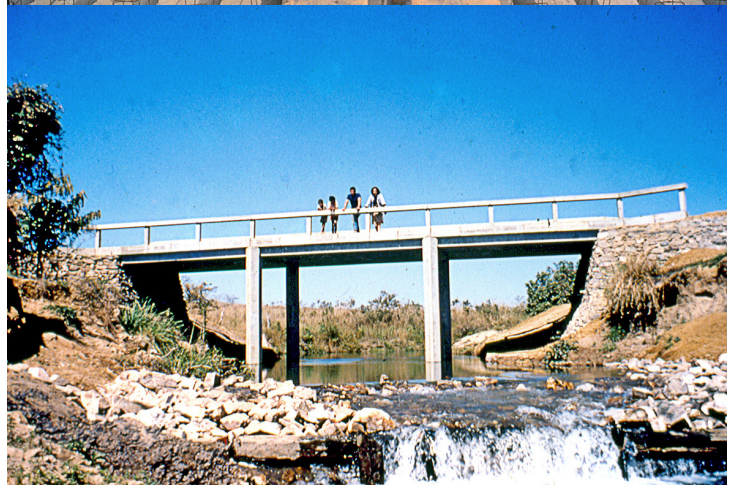
Fig. 3.33 Small bridge (pontilhão) over the Curralinho river in Abadiânia, Lelé, 1983. From top to bottom: initial sketches, the bridge deck’s assembly, and the final result. Arquivo João Filgueiras Lima, Salvador
