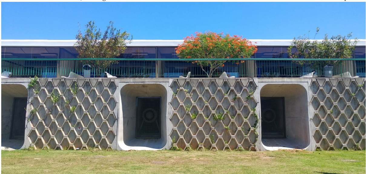
Fig. 1.33 Technical galleries/foundation of the Sarah hospital in Salvador. João Filgueiras Lima, Salvador, 1991. Photograph by Akemi Tahara, 2017
