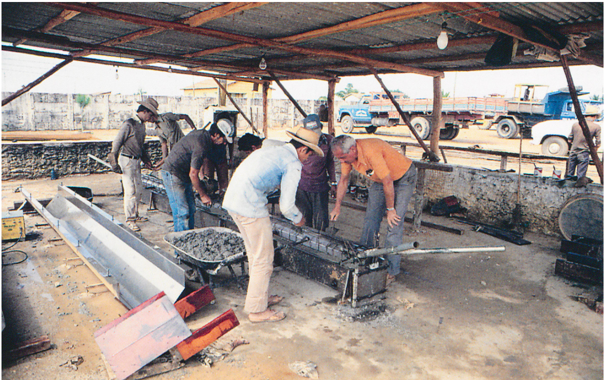
Fig. 3.26 Lelé (on the right) oversees the precast procedure of a rib unity of the bridge deck in Abadiânia, 1983. Argamassa pouring phase in the metallic formwork. Arquivo João Filgueiras Lima, Salvador
