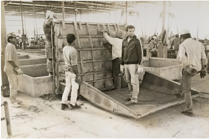
Fig. 2.96 The CIAC's sun canopy in argamassa armada just demolded from the metallic formwork. Brasília, 1991. Arquivo Kristian Schiel, Brasília
