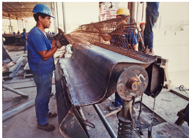
Fig. 2.73 A bench’s metallic formwork being set. Lelé and Mariano Casañas, 1984. Arquivo João Filgueiras Lima
