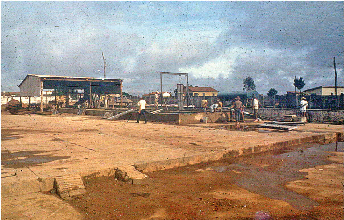
Fig. 3.34 Second factory in Abadiânia. The plant was installed to produce all the precast elements of the transitory school prototype. Lelé, 1984. Arquivo João Filgueiras Lima, Salvador
