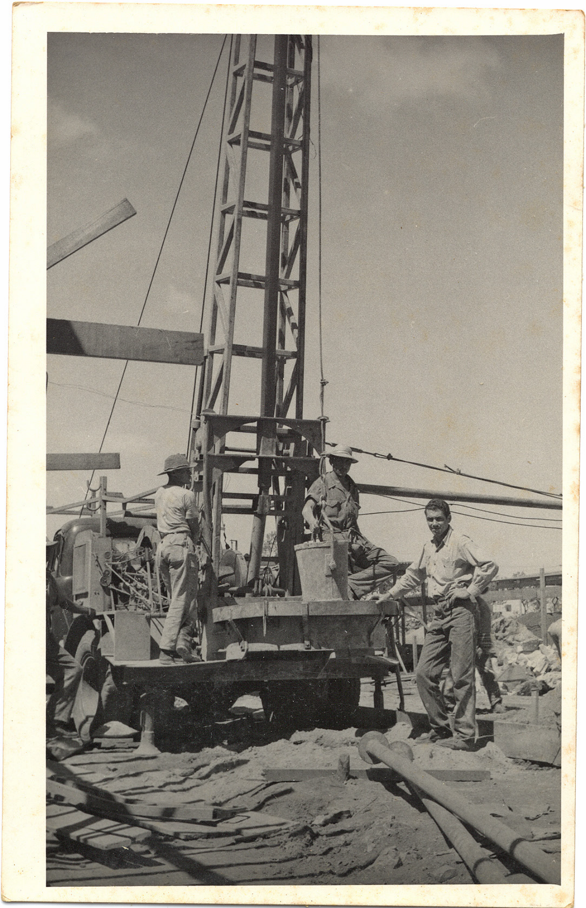
Fig. 1.i Workers on the building site of the first Superquadra (SQS 108) erected in Brasília, 1957. Lelé is the one on the right. Arquivo João Filgueiras Lima, Salvador
