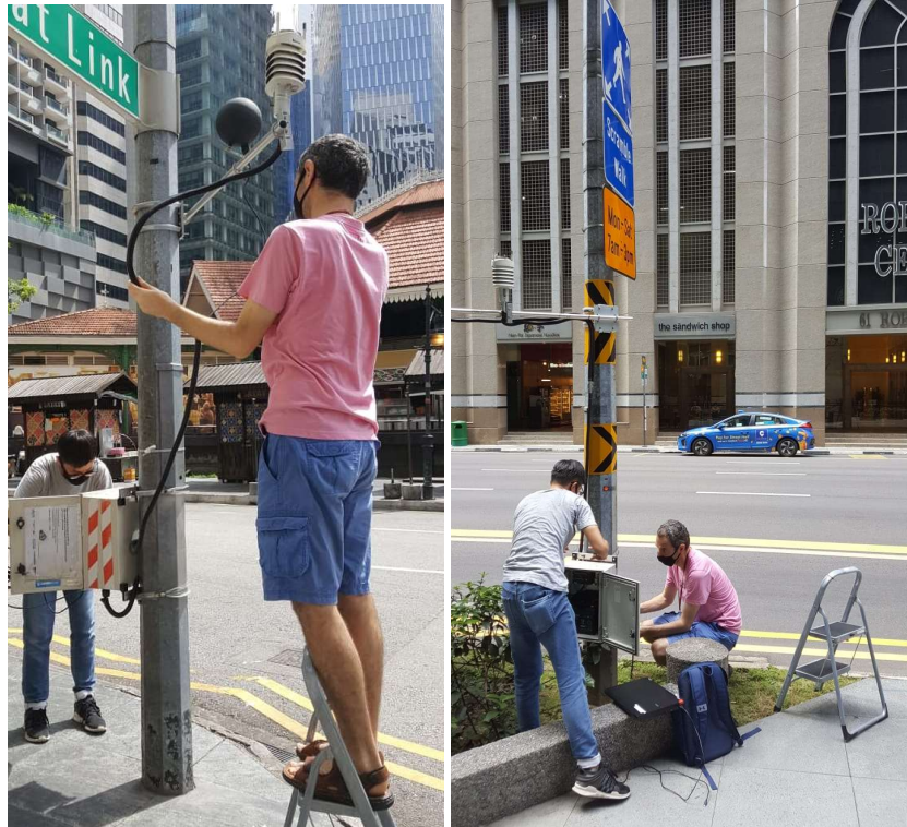
Figure 3: Installation of local weather stations in the Central Business District of Singapore to measure the local climatic conditions (2 m above ground) (Image: Cooling Singapore, 2020)
