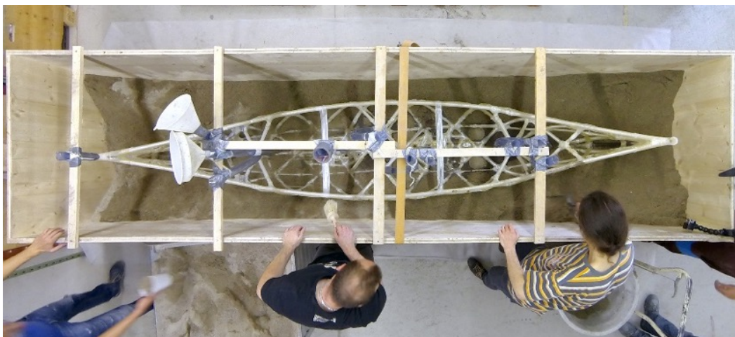
Figure 5.15: The canoe formwork was placed in a simple box that was simultaneously being filled with sand while concrete was being cast inside the formwork (dbt, PCBM, ETH Zürich, 2017)
