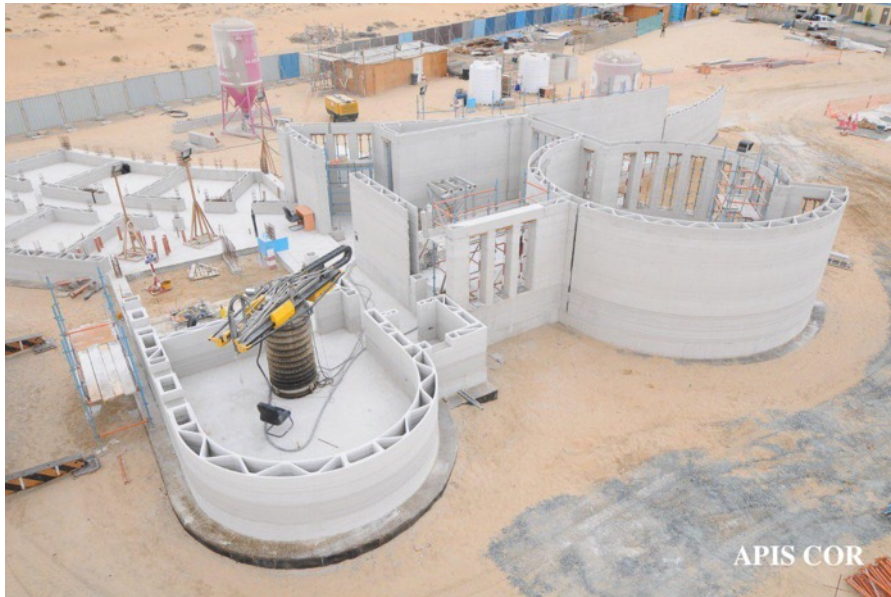
Figure 2.10: Dubai administrative building produced by concrete extrusion 3D printing. (Photo: Apis Cor, 2019)
