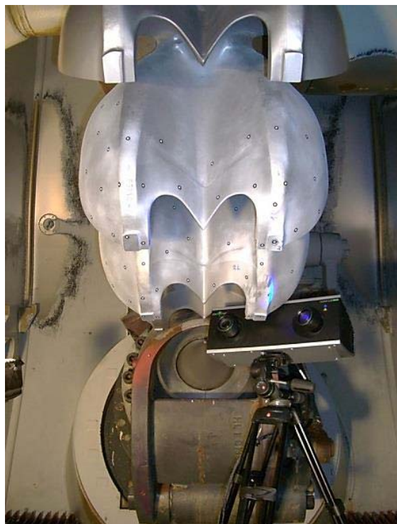
Figure 3-11 Surveying of the current geometry of selected Pelton runner buckets inside the turbine housing in HPP Fieschertal (Abgottspon et al. 2016a).
