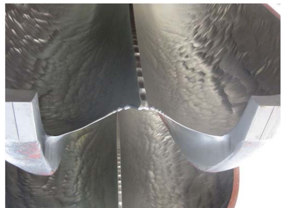
Figure 1-2 Example of a Pelton turbine with damages mainly due to hydro-abrasive erosion (at display at Emosson dam, Switzerland).
