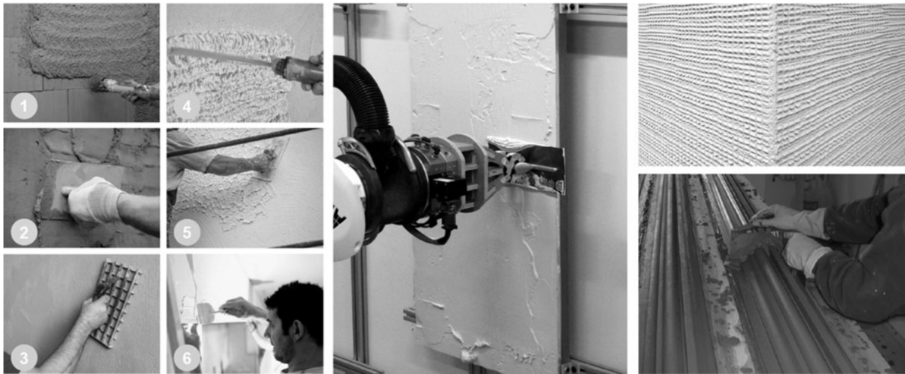
FIG. 1. Left : Steps of a typical plastering process: (1), (2), (3) application of the base coat; (4), (5) application of the top coat; and (6) application of the smooth coat. Middle : Robotic arm with a smoothing trowel, imitating one step of the manual procedure, Bard et al. 2 Top right : Textural detail from surface finishing, Spiro et al. 1 Bottom right : Plasterer with a running mold, taken from https://www.plasterworkspecialist.com .
