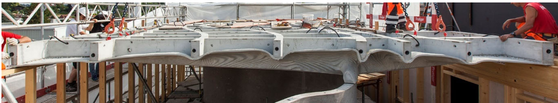
Fig. 2. A section through the Smart Slab shows the variable-height post-tensioned upstand ribs, as well as the ultra-thin interstitial concrete surface.
