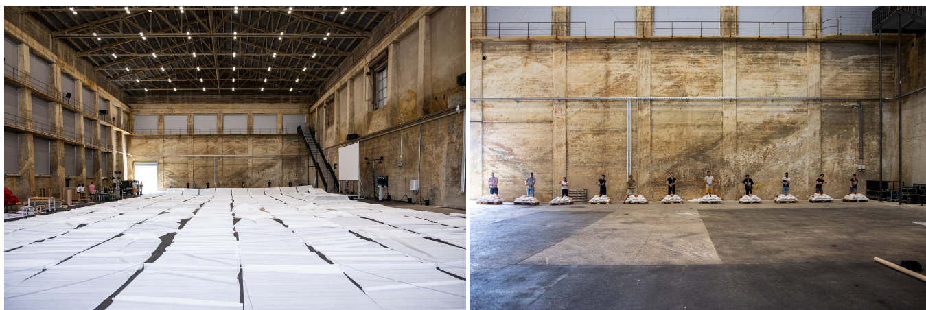
Figure 15. The 10 fabric strips were first unrolled on the ground and connected to the cables (a). The entire system was later lifted into the final position through a set of hand-operable winches located at the ground level (b). Photos by Shuaizhong Wang.
