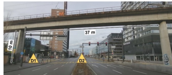
Figure 4. Investigated bridge segment and scanner positions at both measurement days (D1 and D2).
